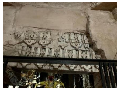
Photo 19: Right jamb of door no.2
